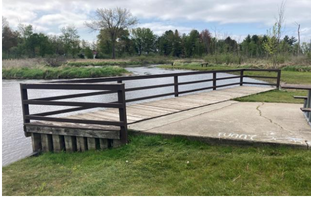
Handrail Does Not Meet ADA Standards
